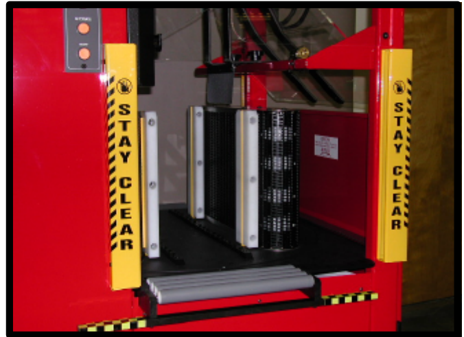
A Light Curtain installed on a QUIPP 400 Stacker, light source to the right and receiver unit to the left. Note the open configuration and the absence of exposed cabling.
